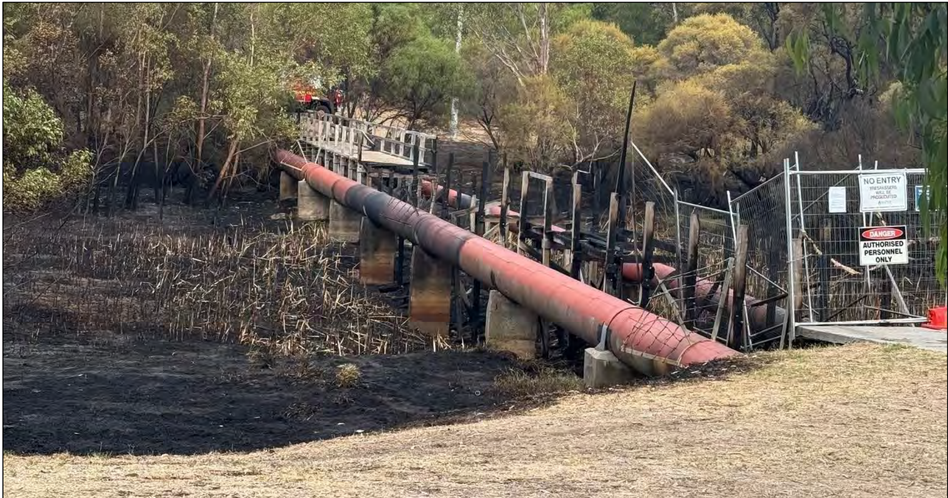
Figure 2 – Damage to the bridge, water and sewer mains caused by the fire
