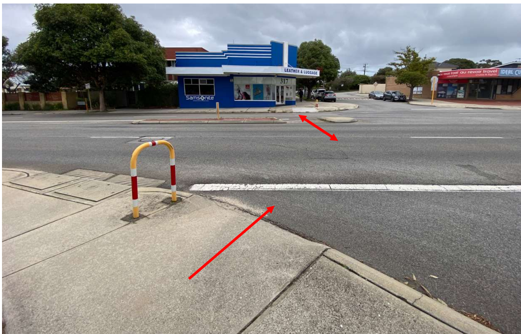
Finding 2.7 – Pedestrian gap not aligned at 90 degrees to adjacent ramp potential to lead visually impaired to Adair Parade. Pedestrian ramp grade not at 90 degrees to gap leading wheelchairs away from adjacent gap on Walcott Street. No TGSIs.
