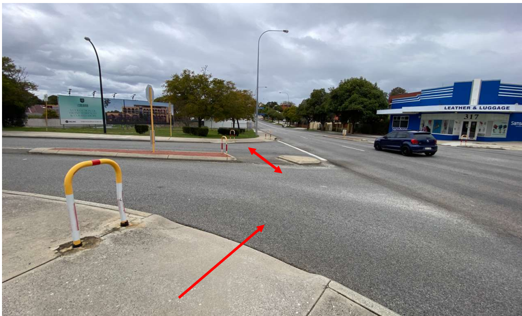
Finding 2.7 – Pedestrian gap not aligned at 90 degrees to adjacent ramp potential to lead visually impaired to Walcott Street. Pedestrian ramp grade not at 90 degrees to gap leading wheelchairs towards Walcott Street. No TGSIs.
